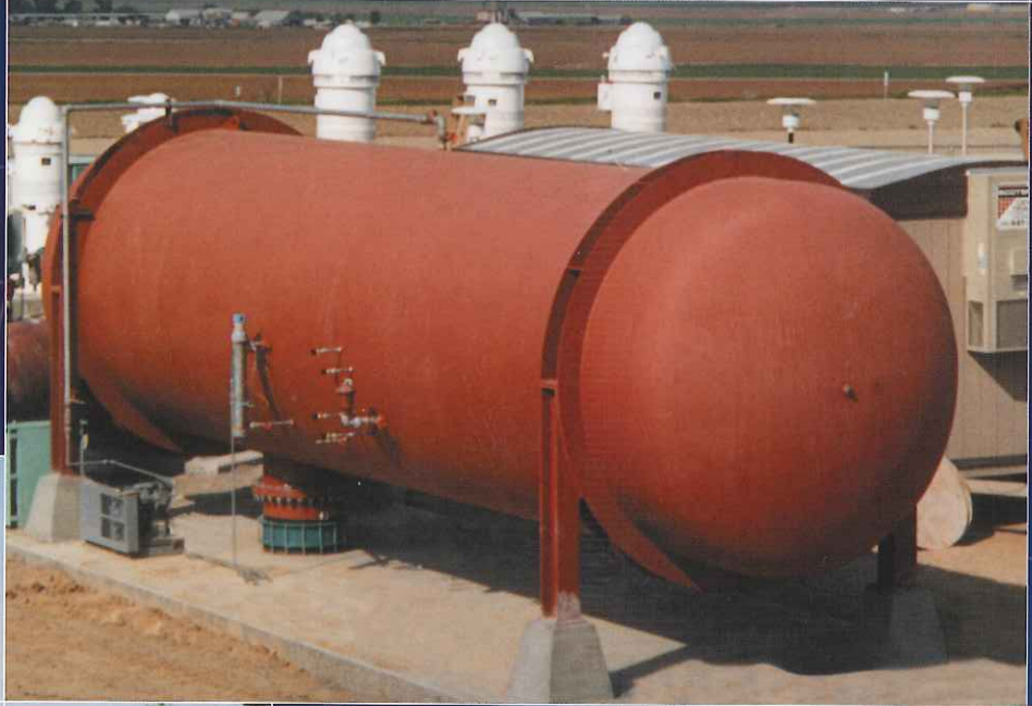
Surge Tank 21,000 gallon capacity, with a working pressure of 150 PSI
