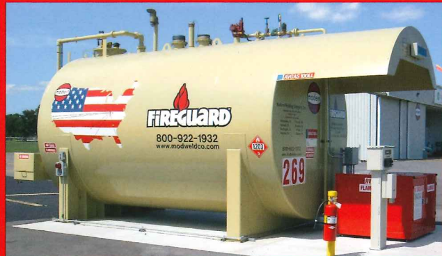
10,000 Gallon Capacity AVGAS Storage
